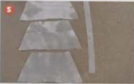
PHOTO 5: The glass-cloth pieces are cut to size (Some of the strips are needed).
