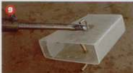
PHOTO 9: Small pieces of fibreglass are soldered to the pipes at the points where they pass through the tank.
